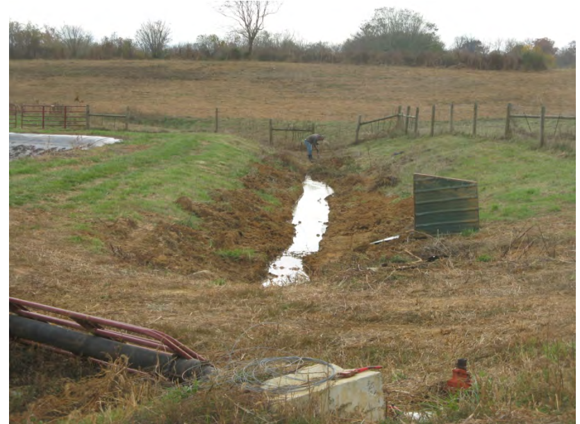
drainage ditch ponded below culvert
