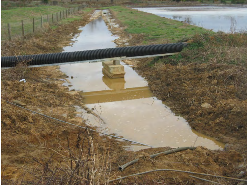
Stormwater ponded behind culvert
