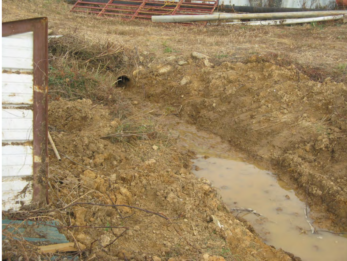
culvert that needs to be replaced
