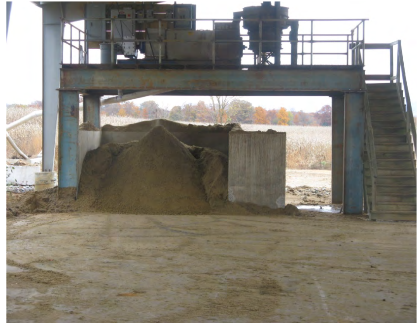
separator relocated and in operation
