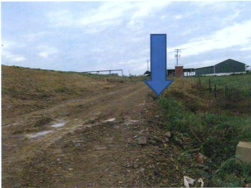
access road to manure storage pits graded – silt fence to be installed (arrow)to direct stormwater away from monitoring well #1
