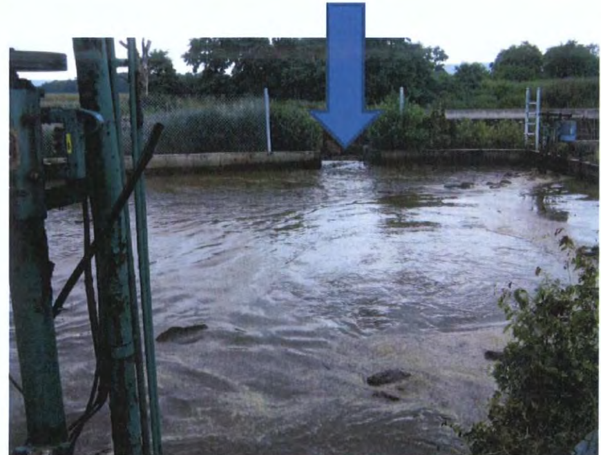
Spill way from reception pit to settling basin
