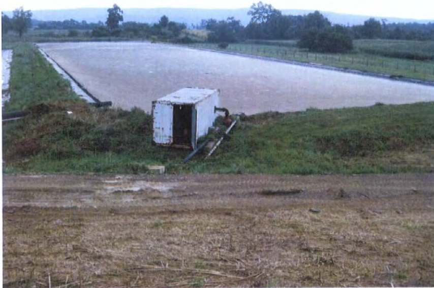
Pump house for pumping flush water To flush tanks from manure pit #1 Also, the manure storage pit is at capacity -18 inch freeboard
