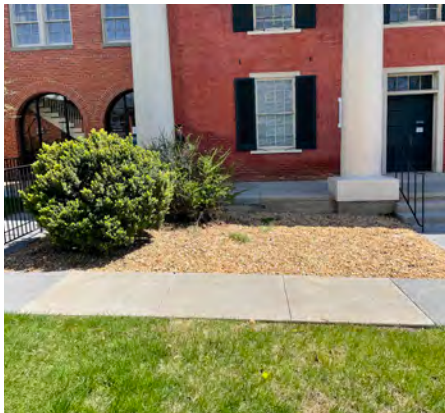
Planting beds at the front of the Old Courthouse and around the northeast side have minimal planting and gravel fill that spills onto the walking surfaces.
