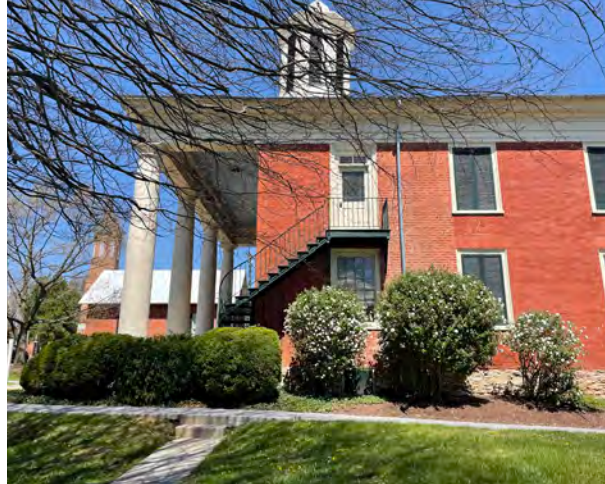
Against the Old Courthouse building, a variety of large shrubs block the view of the building, trap moisture behind the walls, and impede foot traffic along the narrow sidewalk.
