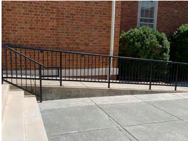
The ramp connecting the ADA parking spaces at the southeast to the New Courthouse building has a sloping sidewalk with one section steeper than required by ADA.
