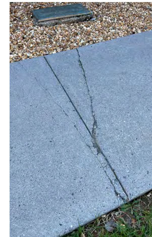
Pavement cracking/uneven settling
