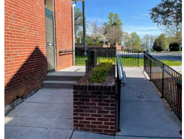
The ramp connecting the northwest vehicle drop-off with the Old Courthouse building has a slope steeper than required by ADA.
