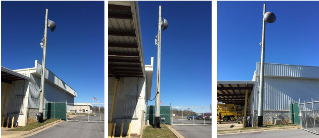
Monopole Cell Tower (Typical)
