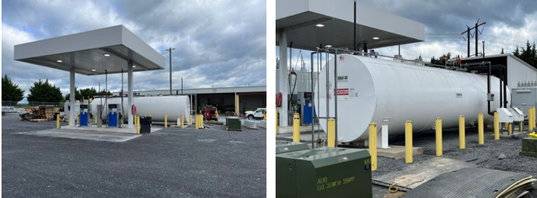
Fleet Fuel Area with AboveGround Storage Tank (Typical)
