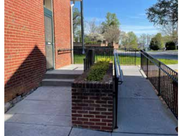
The ramp connecting the northwest vehicle drop-off with the Old Courthouse building has a slope steeper than required by ADA.
