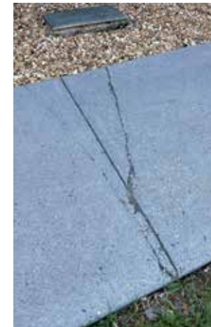
Pavement cracking/uneven settling
