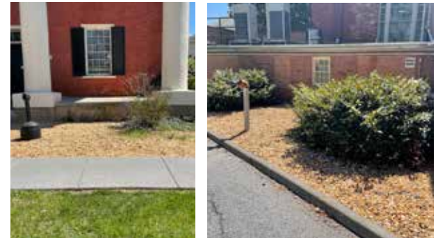
Planting beds in front of the Old Courthouse and extending around the north side of the building have a tan gravel fill and dying plantings.
