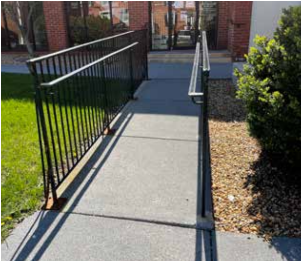
The ramp connecting the N. Church Street sidewalk with the Old Courthouse building has a slope steeper than required by ADA.
