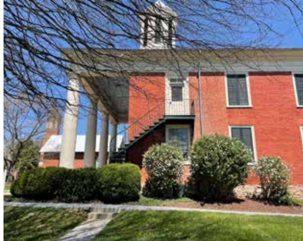
Against the Old Courthouse building, a variety of large shrubs block the view of the building, trap moisture behind the walls, and impede foot traffic along the narrow sidewalk.
