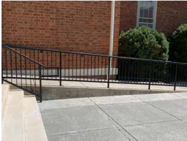
The ramp connecting the ADA parking spaces at the southeast to the New Courthouse building has a sloping sidewalk with one section steeper than required by ADA.
